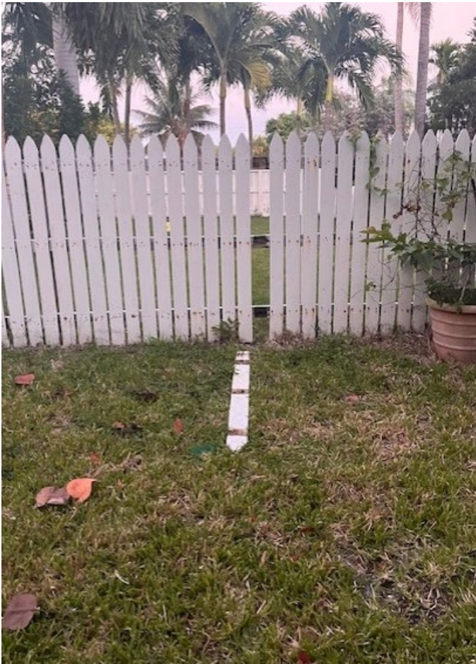
@#69 – HOA Repairs, paint needed. Broken gate opener – This was on the Survey
